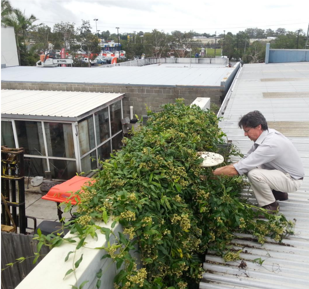
Figure 16. Antenna covered by vegetation at site BEE2 in Queensland, Australia.
