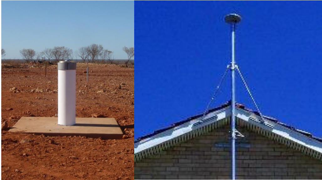
Figure 21. Typical installations of station monument types class A (left) and B (right).
