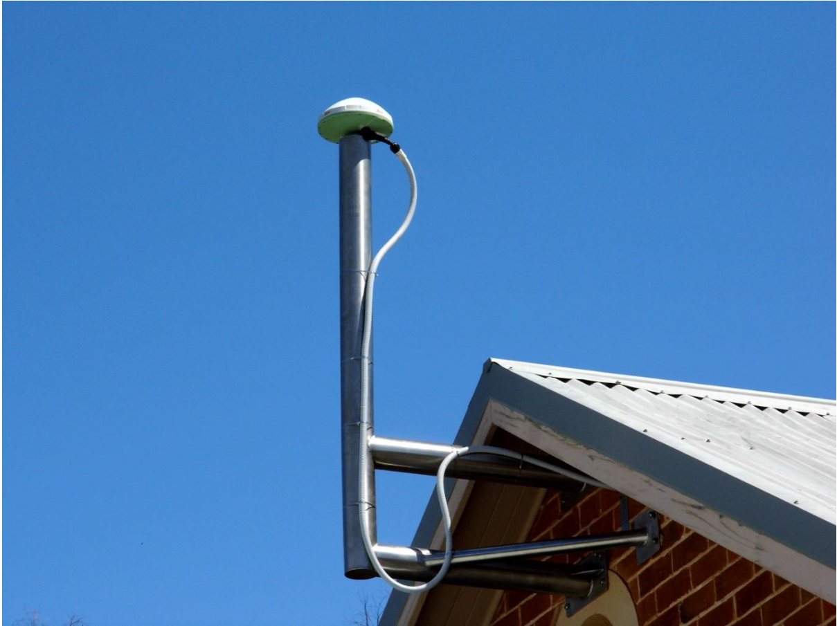
Figure 4. A typical installation of a CORS site attached to a building via a stainless steel mast.
