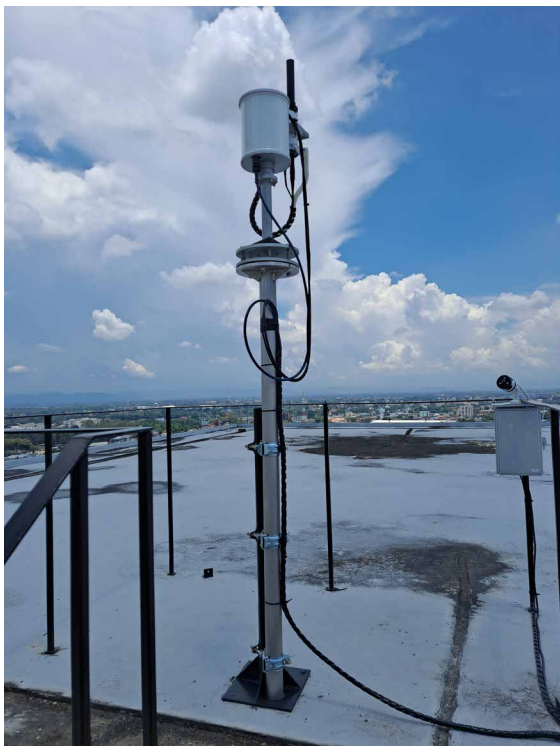
Figure 2.3: Pandora instrument installation on a rooftop of the Chiang Mai Rajabhat University
